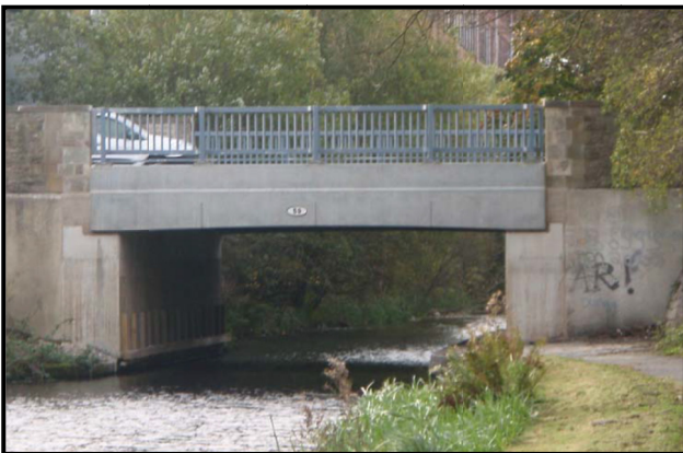
Greater Manchester, UK. The 13 m wide, 9 m long Moss Canal traffic bridge comprises pultruded GFRP double-web beams (DWBs) laid on their sides to act as both a cellular deck and the main longitudinal beams. The fibre type was changed from carbon in the standard DWB to glass for this specific application. This deck was proof-tested under 10 million cycles of local wheel load fatigue at the University of Bristol, supervised by Dr Wendel Sebastian. The DWB deck arrangement weighs 40% of the original deteriorated concrete deck, so the original bridge abutments and foundations were re-used. Designer - SKM Ltd. Main contractor - Askam Construction Ltd. Supplier - Pipex Ltd / Strongwell, 2012.
