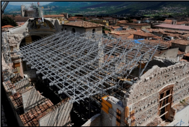
S. Maria Paganica Church, L'Aquila (Italy). Replacing the roof of the church damaged by the earthquake of April 2009. GFRP pultruded members. Designers: prof. Salvatore Russo, ing. Alessandro Adilardi. Contractor: Top Glass S.p.A, Osnago (LC), 2010.
