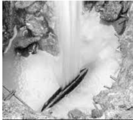
FIGURE 1.1: Longitudinal crack in PE pipe, as reported by Rozental (2009).
