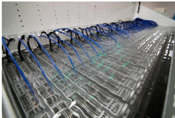
Figure 2.12 Liquid submersion cooling from Green Revolution Cooling (Green Revolution Cooling)
