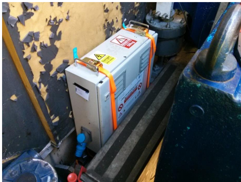
Figure 8.17: CMS2 unit installed within the nacelle
