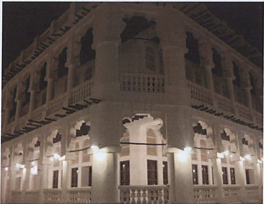
Fig. 13. Traditional decorative gypsum and timber work at Souk Waqif. This is a type of costly decorative work that can be found in traditional wealthy family houses (photographed in 2009).
