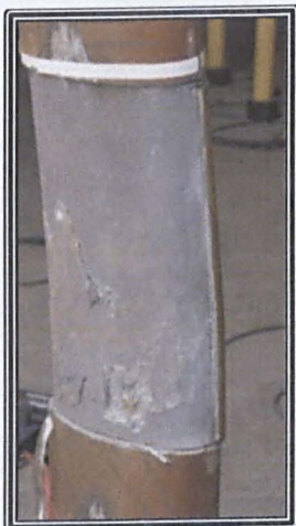
Compression failure of CIII-150-C100
