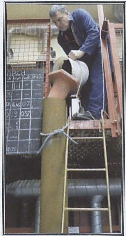
(b) Tube is secured with strings and a cone is used for concrete filling
