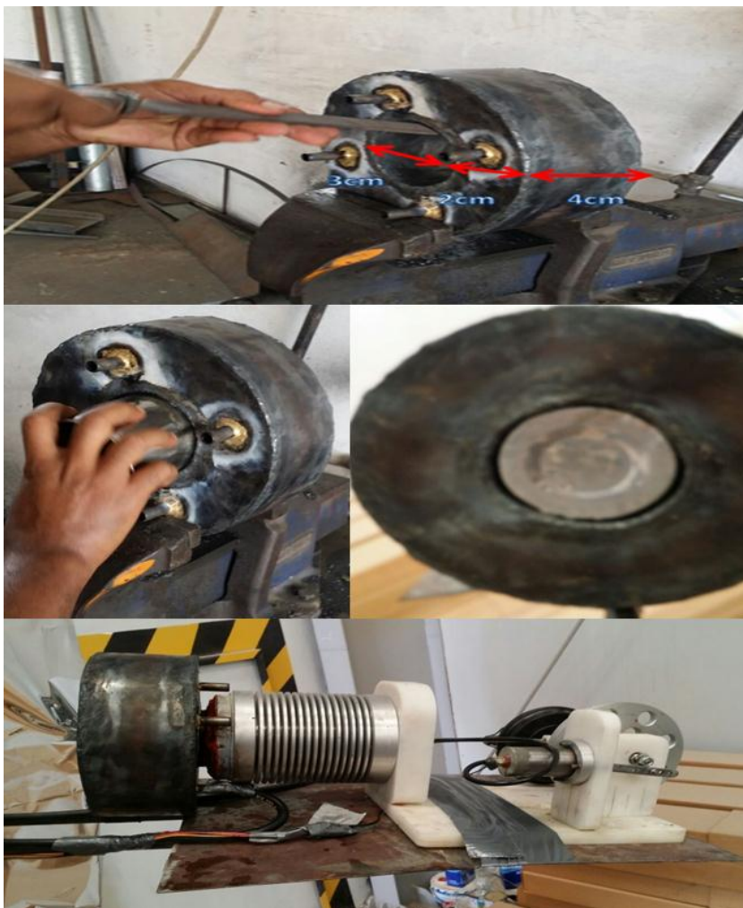
Figure 3.29 Steps of hybrid Stirling engine been installed into cavity receiver
