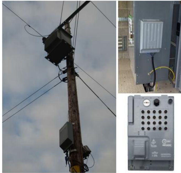
Figure 10: Gridkey MCU 520 substation monitor
