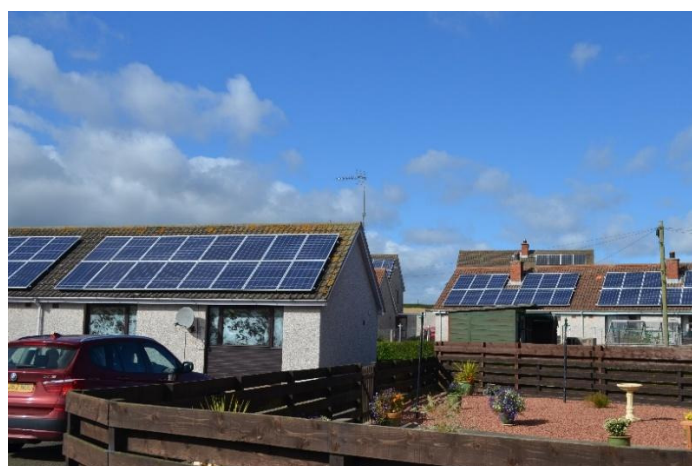
Figure 5: Installed PV panels
