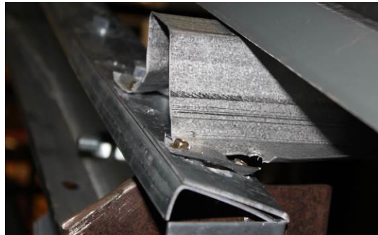
b) Failure of purlin connection and deformation of the gable-frame rafter
