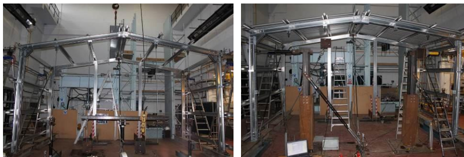
a) Building with no sheeting
