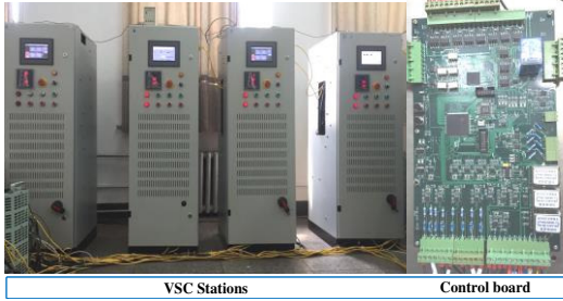
Fig. 15: VSC converters of experimental platform and main driver board of the power converters (right).
