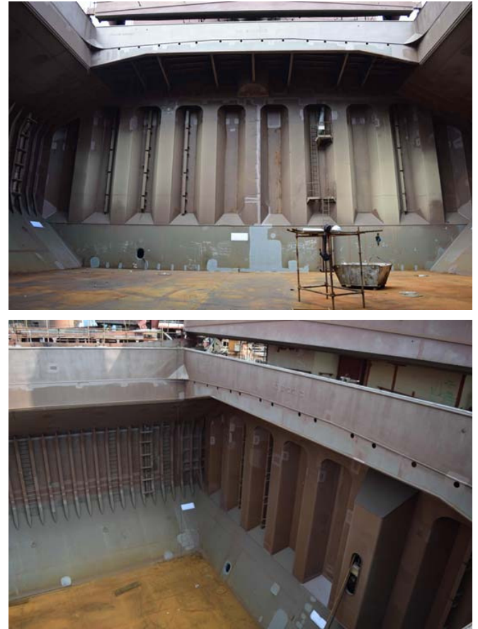
Figure 4. Sample of the field images collected (top) from the location of the tank top and (bottom) deck
