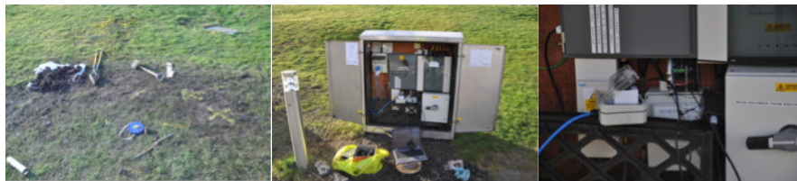
Figure 6: Test site in Falkirk Wheel after the deployment of all subsurface sensor nodes and housing for power supply, getaway and hub.
