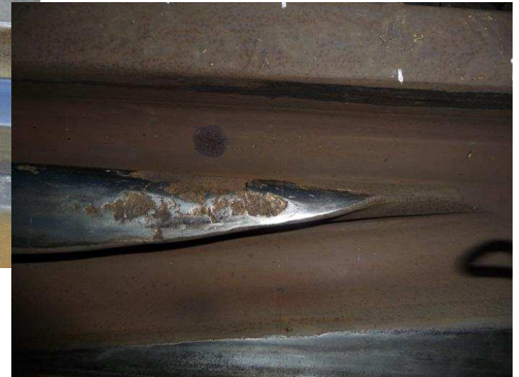
Spalling & plastic deformation of crossing nose
