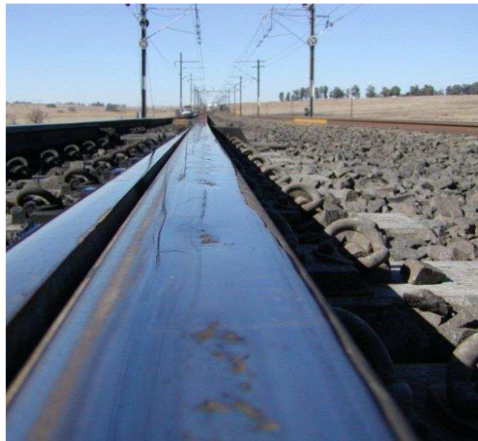
Spalling of stock rail
