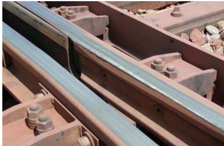
Lipping of switch/stock rails
