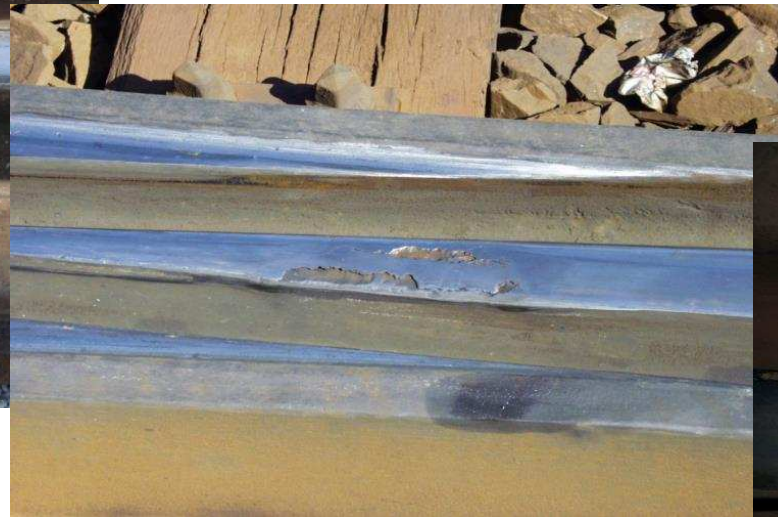
Spalling of crossings
