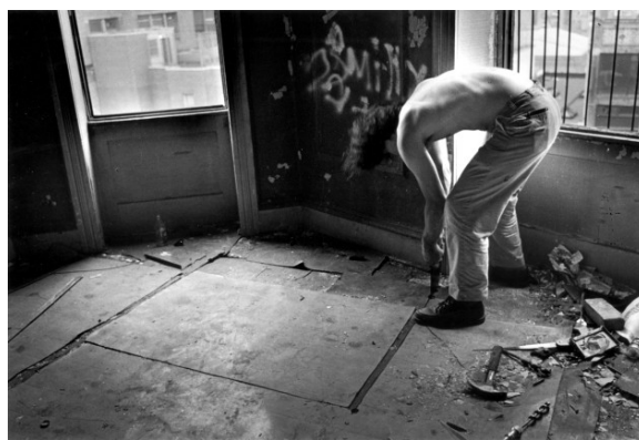
[Fig 21: Matta-Clark, G. (1972) Building cuts . Photograph [Online]. Available at: http://artsdocuments.blogspot.co.uk/2010/10/gordon-matta-clark.html [Accessed 13 Mar 2014].
