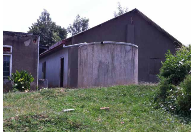
Rain water tank supplies water for 1,100 students
