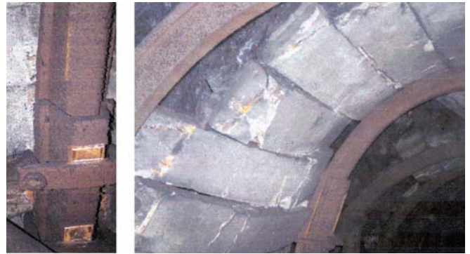
Figure 5. The displacement in the yielding steel sets and deformation in struts on the beneath level of the fractural zone (level 2200 m).
