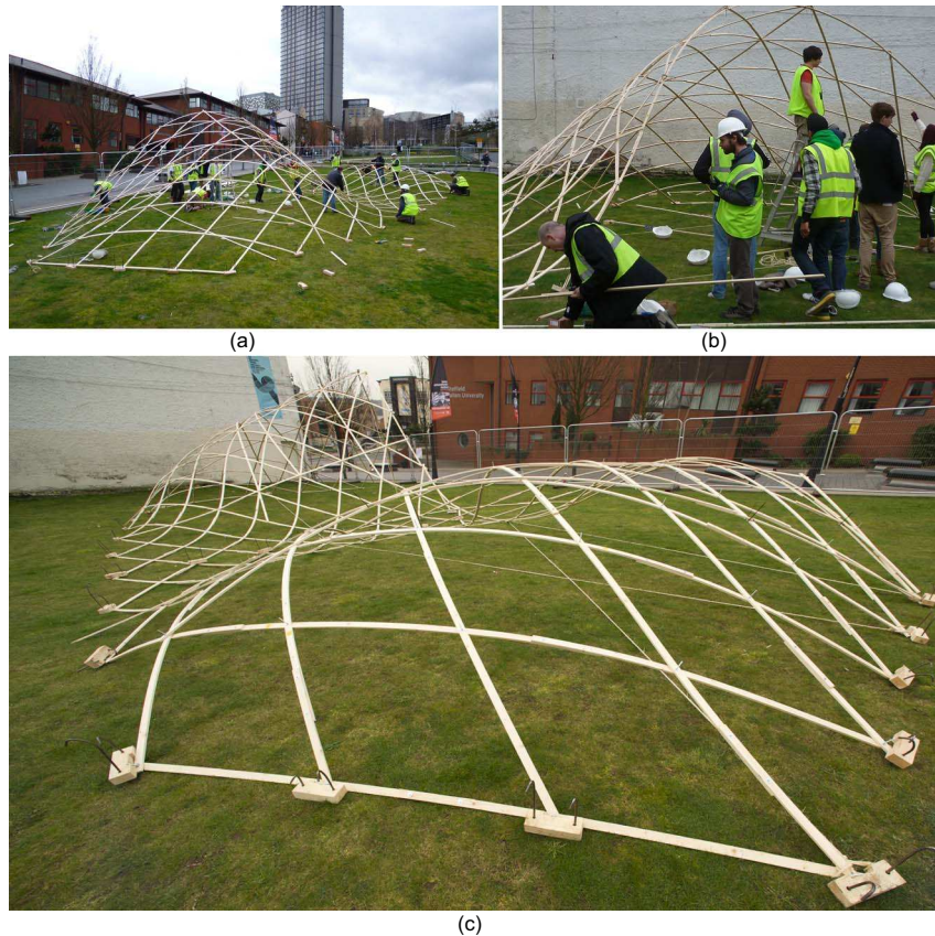
Figure 10. (a): The geometry of the structure was stabilised by bracing and triangulation. (b): The swells nearing completion. (c) The swells on display at Sheffield City Centre
