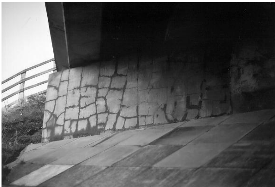
Figure 10: Restrained shrinkage cracking in repair patch. E_{rm} < E_{sub} .
