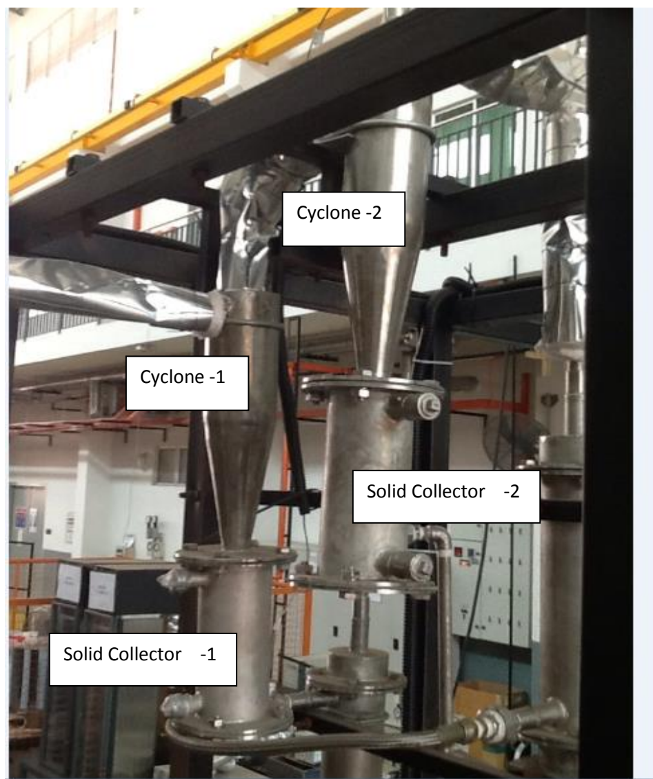
Figure 3-7: Picture of cyclone separators with solid collectors
