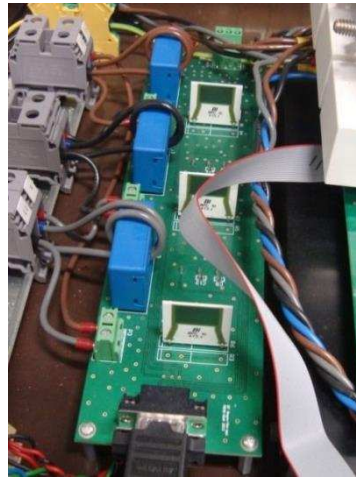
Fig. 7.21 Supply voltage/current measurement board (voltage transducers are underneath).
