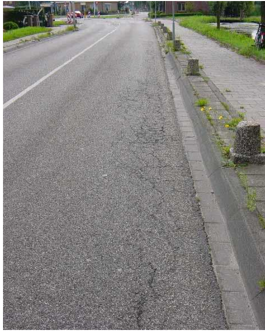
(a) Longitudinal and Alligator Cracking
