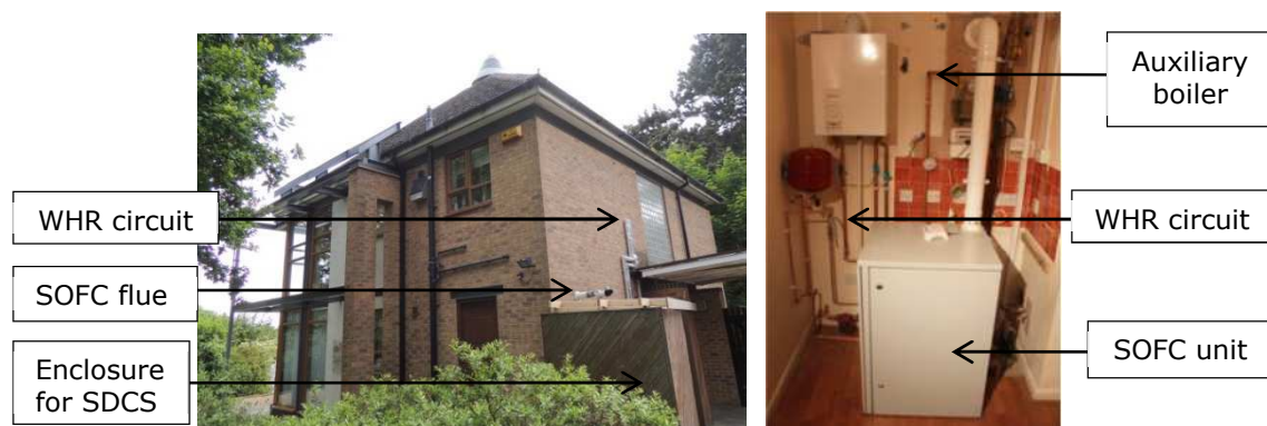
Figure 7-1 BlueGEN SOFC CHP system installed at The University of Nottingham
