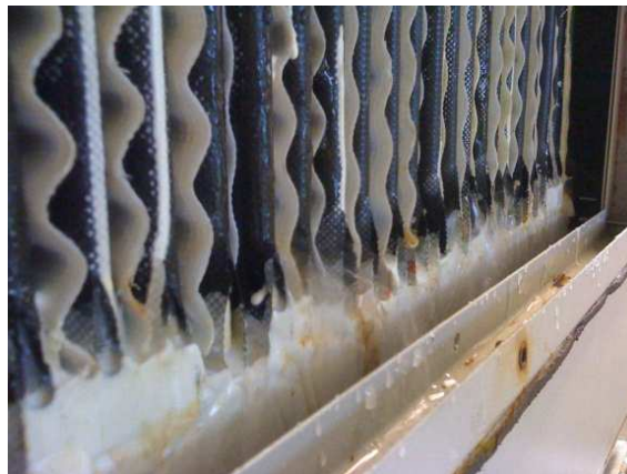
Figure 5-11 Dehumidifier HMX leakage in the IDCS
