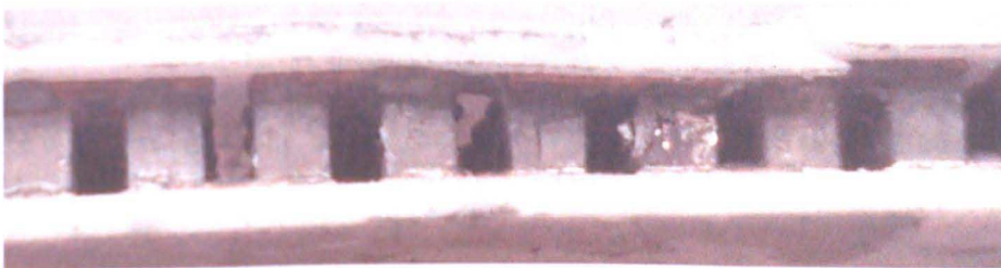
Figure 5-4 Module damages caused by uneven and excessive pressure load
