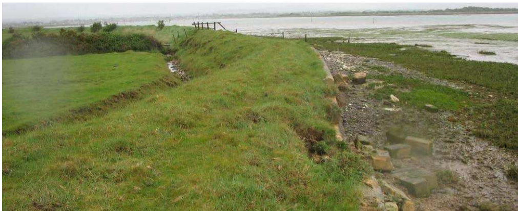
Figure 4-17 Concrete blockwork facing collapse permitting erosion of clay bank
