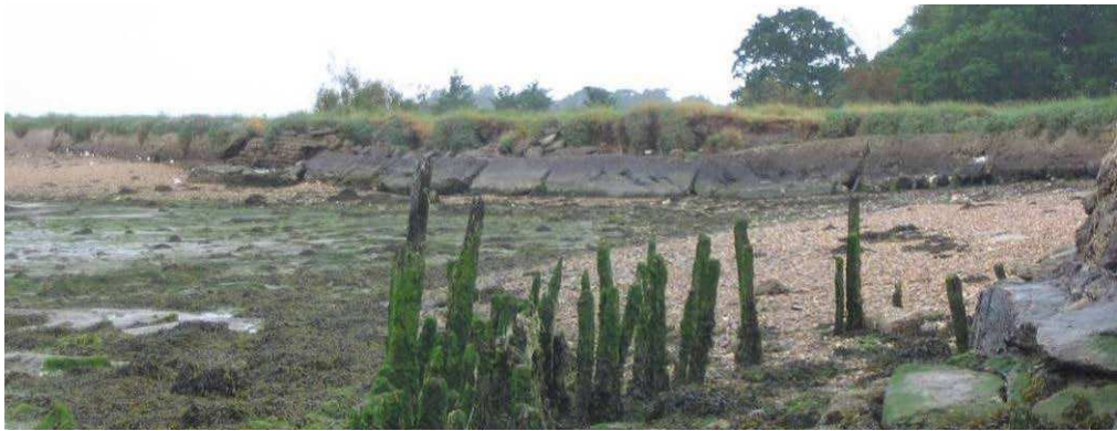
Figure 4-16 Example of collapsed concrete wall (mid picture) and bank erosion above
