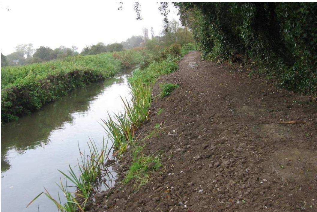
Figure 4-6 (a) Installing coir rolls at base of bank to provide stabilised toe to (b) new bank slope and encourage water line vegetation, September 2008 (Courtesy Hanneys Flood Group)
