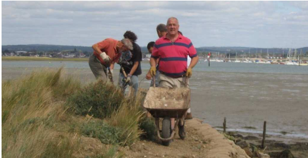
Figure 4-24 Moving and placing clay fill to make up crest of sea wall, 31 August 2009
