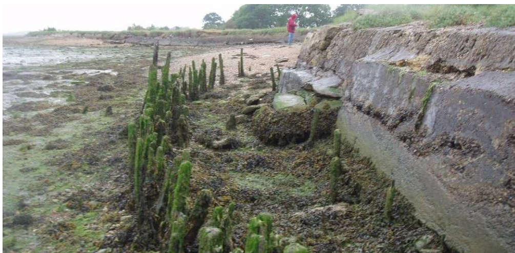
Figure 4-14 Example of mass concrete wall with timber stakes exposed by eroded beach
