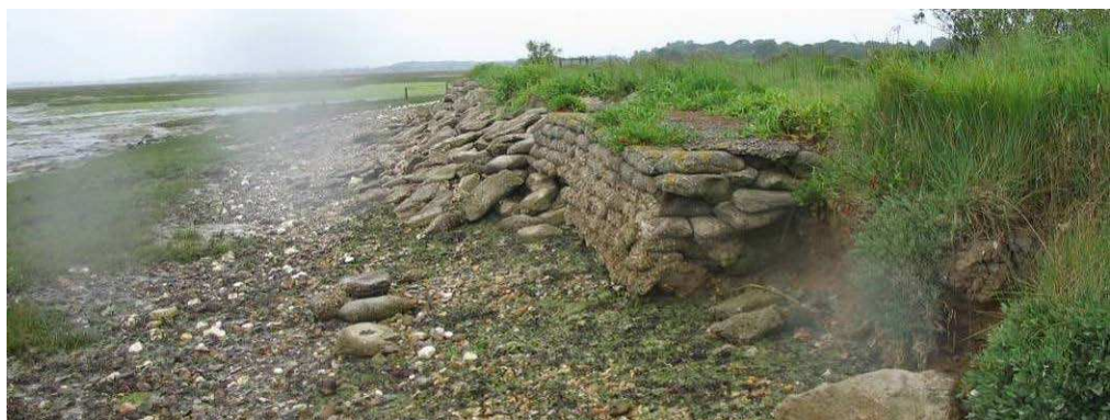
Figure 4-18 Example of existing concrete bagwork walling, including collapsed section in rearground and eroded bank in foreground
