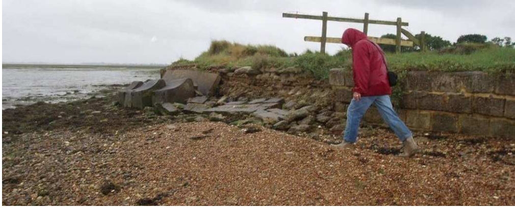
Figure 4-15 Example of collapsed concrete blockwork wall facing.
