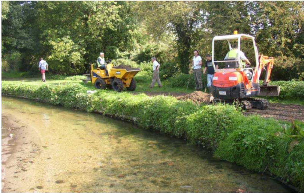
Figure 4-5 Letcombe Brook, showing commencement of low bund construction by Hanneys Flood Group, September 2008 (Note drop in water level compared with previous figure following weed clearance) (Courtesy EA)
