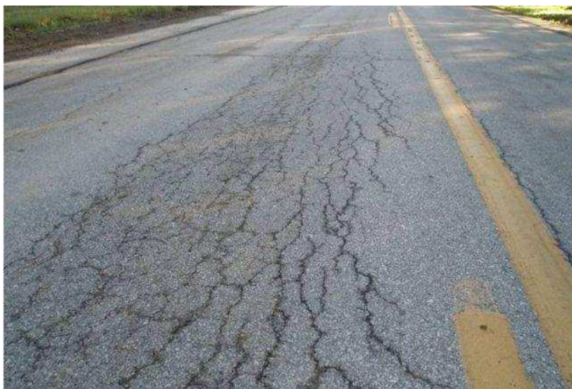
Figure 2.7: Fatigue cracking in practical engineering (Fatigue cracking, 2015)
