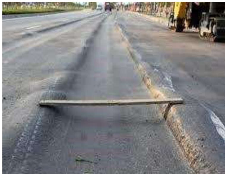
Figure 2.9: Rutting in practical engineering (Quang, 2014)
