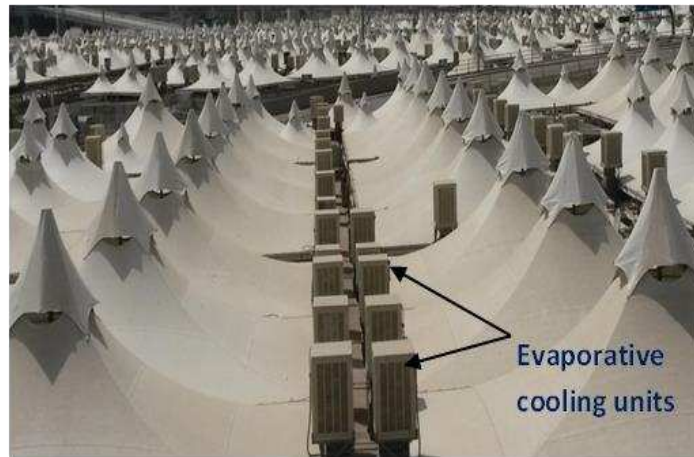
Figure 8.1 Roof top mounted evaporative cooler for cooling in pilgrims' accommodations
