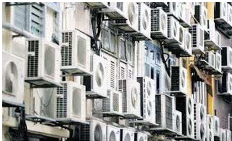
Figure 3.14 Air conditioning installed in residential building, Saudi Arabia [46]
