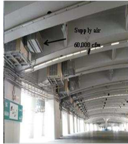
(b) Evaporative cooler unit
