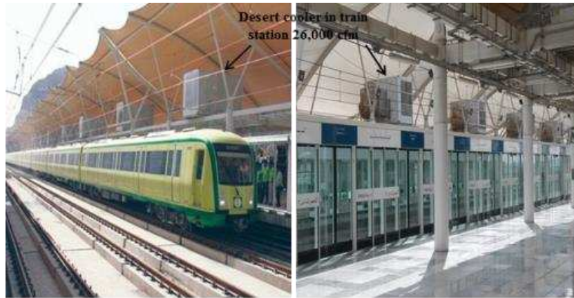
Figure 8.7 Evaporative cooling units in the train station
