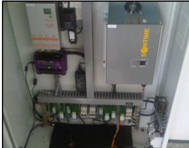
Figure 132 Power Electronics used in Solar Cabin
