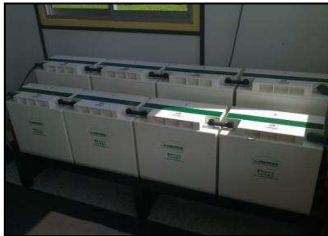
Figure 133 Batteries used in Solar Cabin
