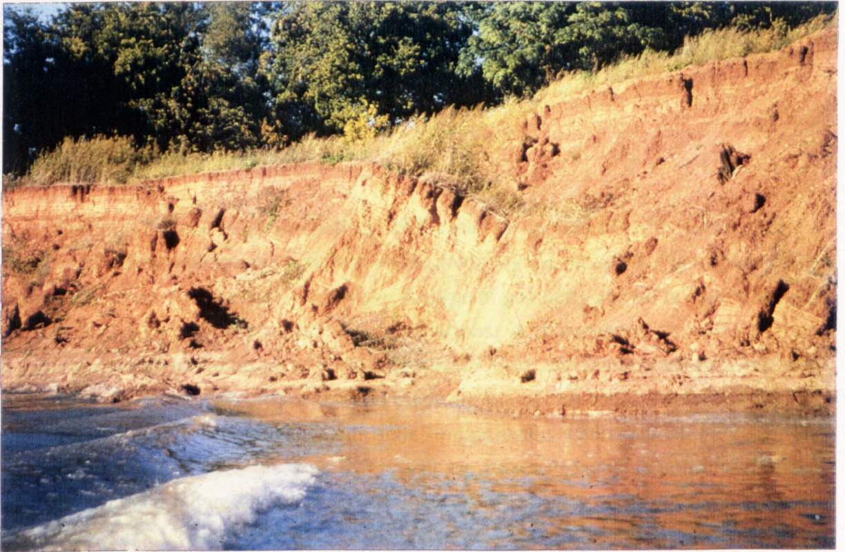
Plate 3.1 Geometry of Rotational Slip Failure on the Red River, Louisiana
