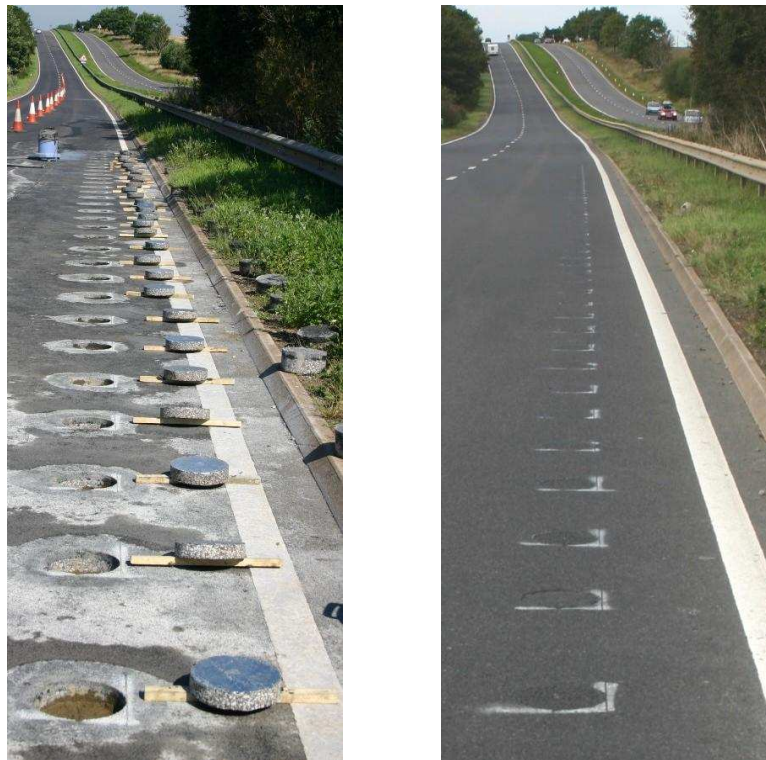
Figure 5.1 Asphalt discs in lane 2 of the A5 sites, about to be installed (left) and shortly after installation (right)
