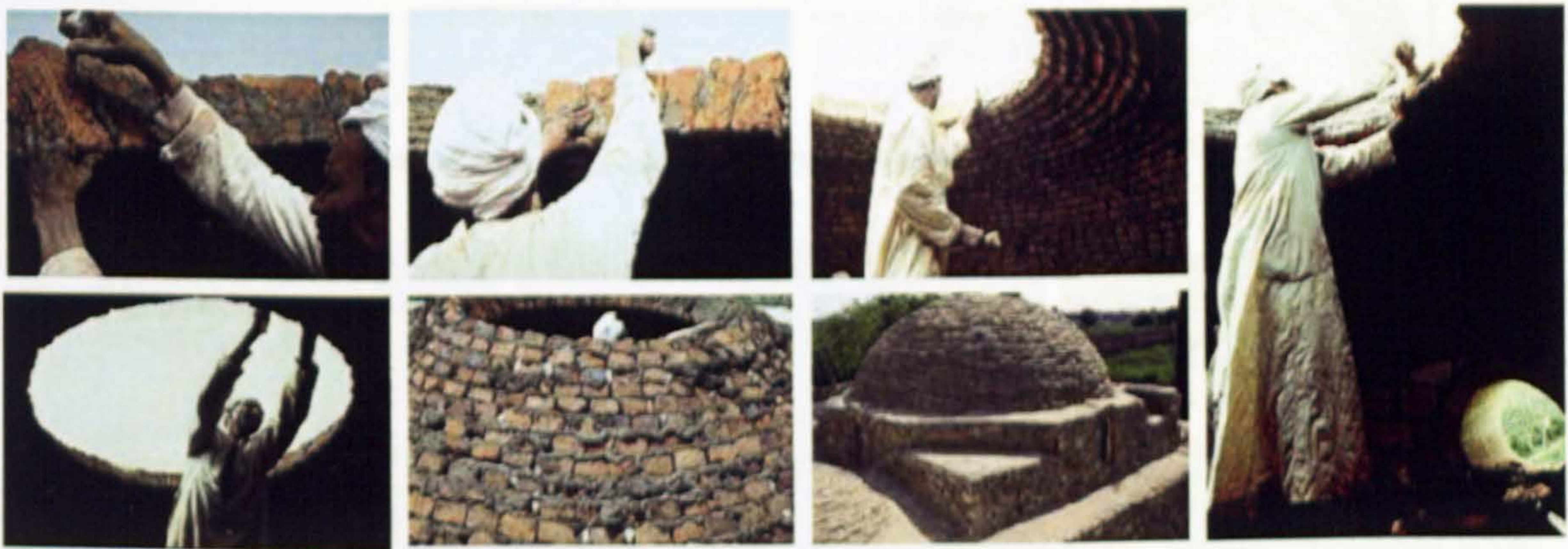
Figure 4-7 The traditional Process of Erecting Woodless Mud Bricks' Domes Source: ArchNet Digital Library [13]
