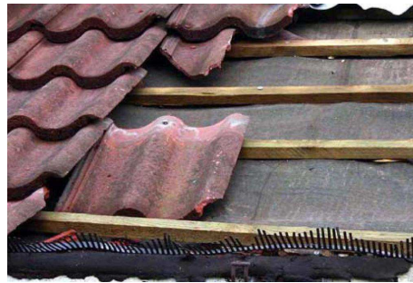
Figure 1.3: Photo from a damaged roof in Birmingham showing the typical UK roofing tile with nailing only at the top making bottom uplift easy (Marshall and Robinson, 2006).
