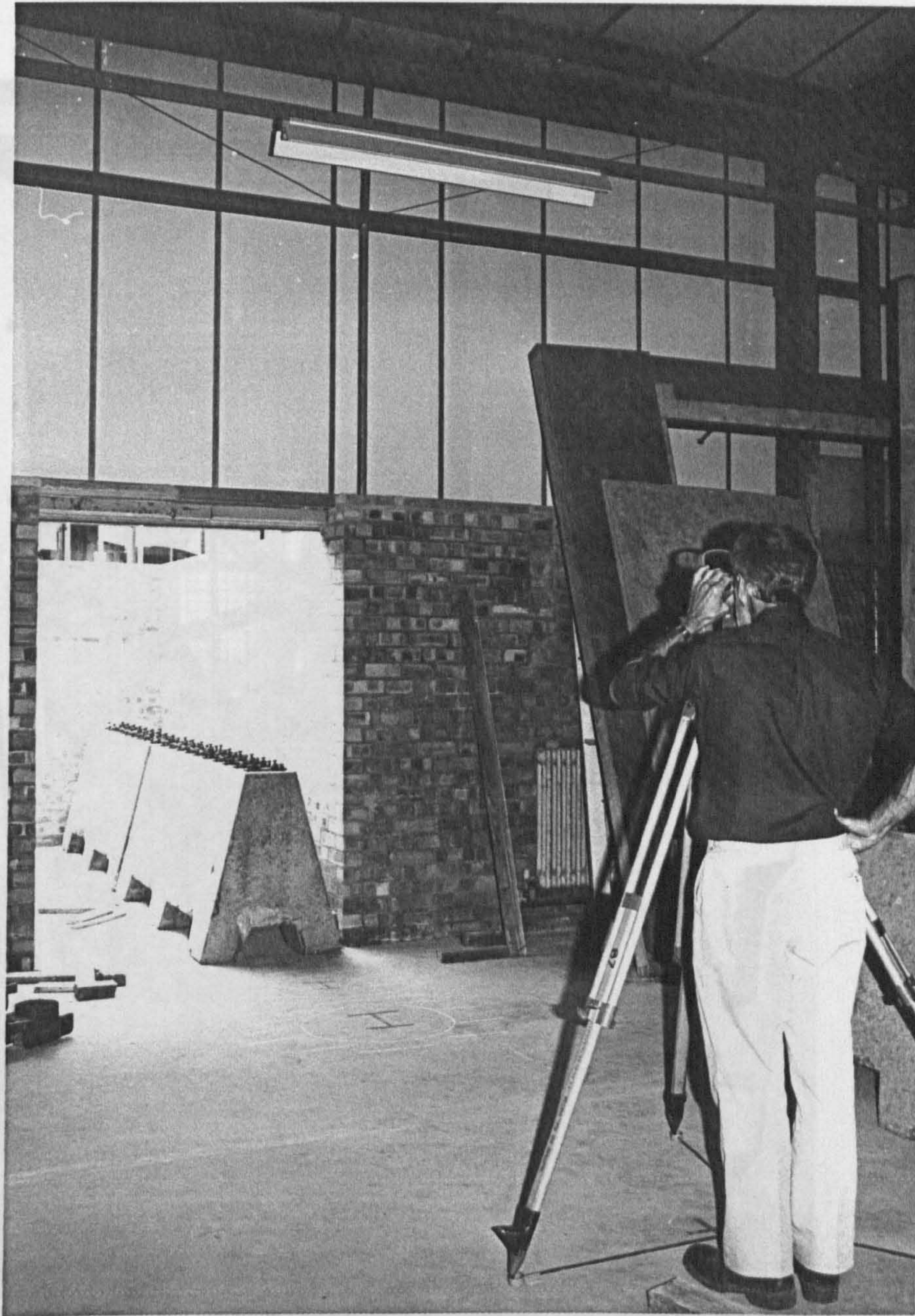
Installation of the working section floor. The moving model rig track (I beam) is shown installed on the concrete blocks. The flow collector section, fan and motor are from the original tunnel.
