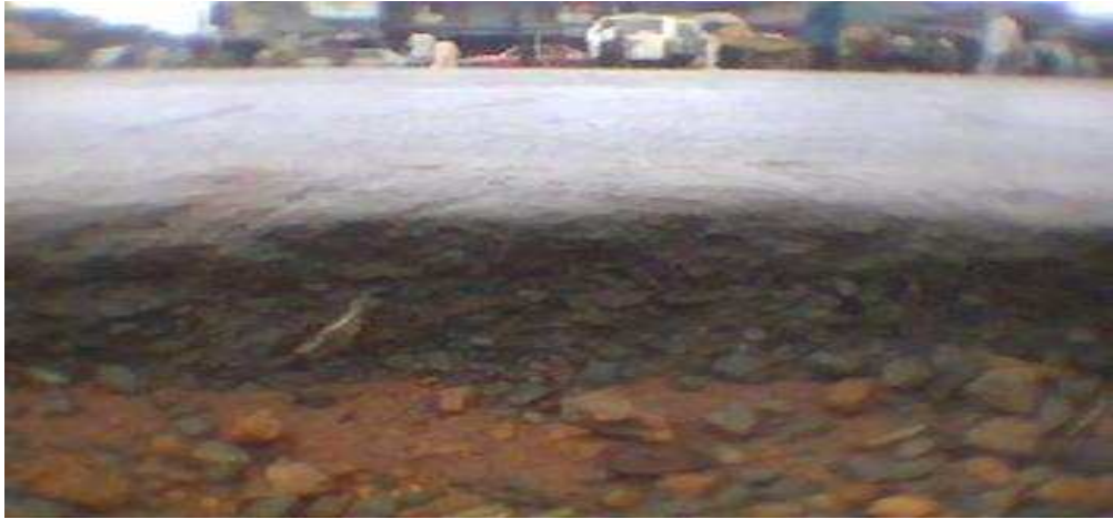
Figure 2.4b: Very Thick Asphalt Layer Due to Several Overlays in Ibadan, Nigeria
