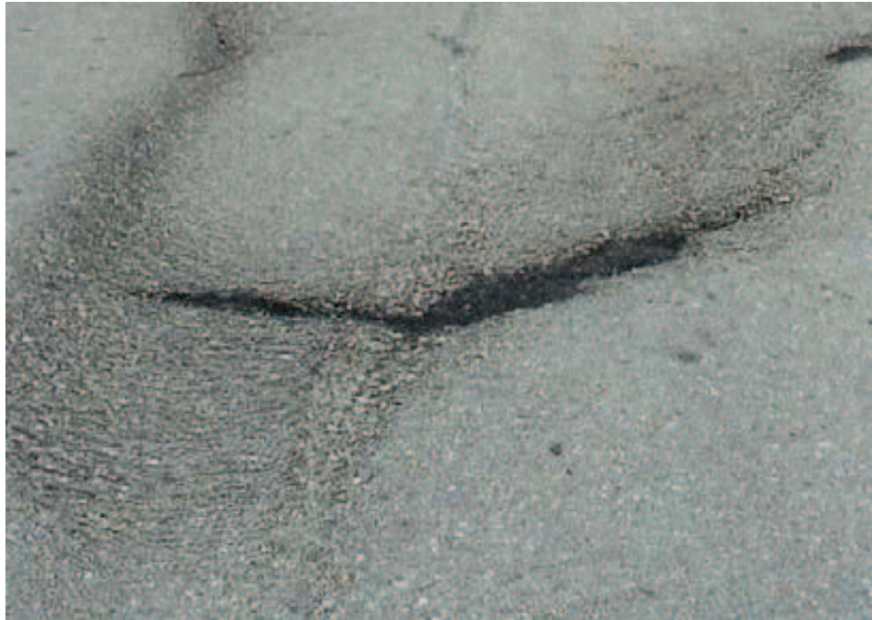
Figure 2.19 – Crescent shaped slippage crack (From West et al. ,1987)
