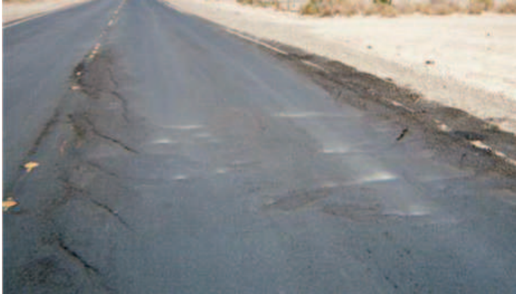
Figure 2.4 – Premature slippage failure on an overlay project in Nevada, USA (Charmot et al. , 2005)
