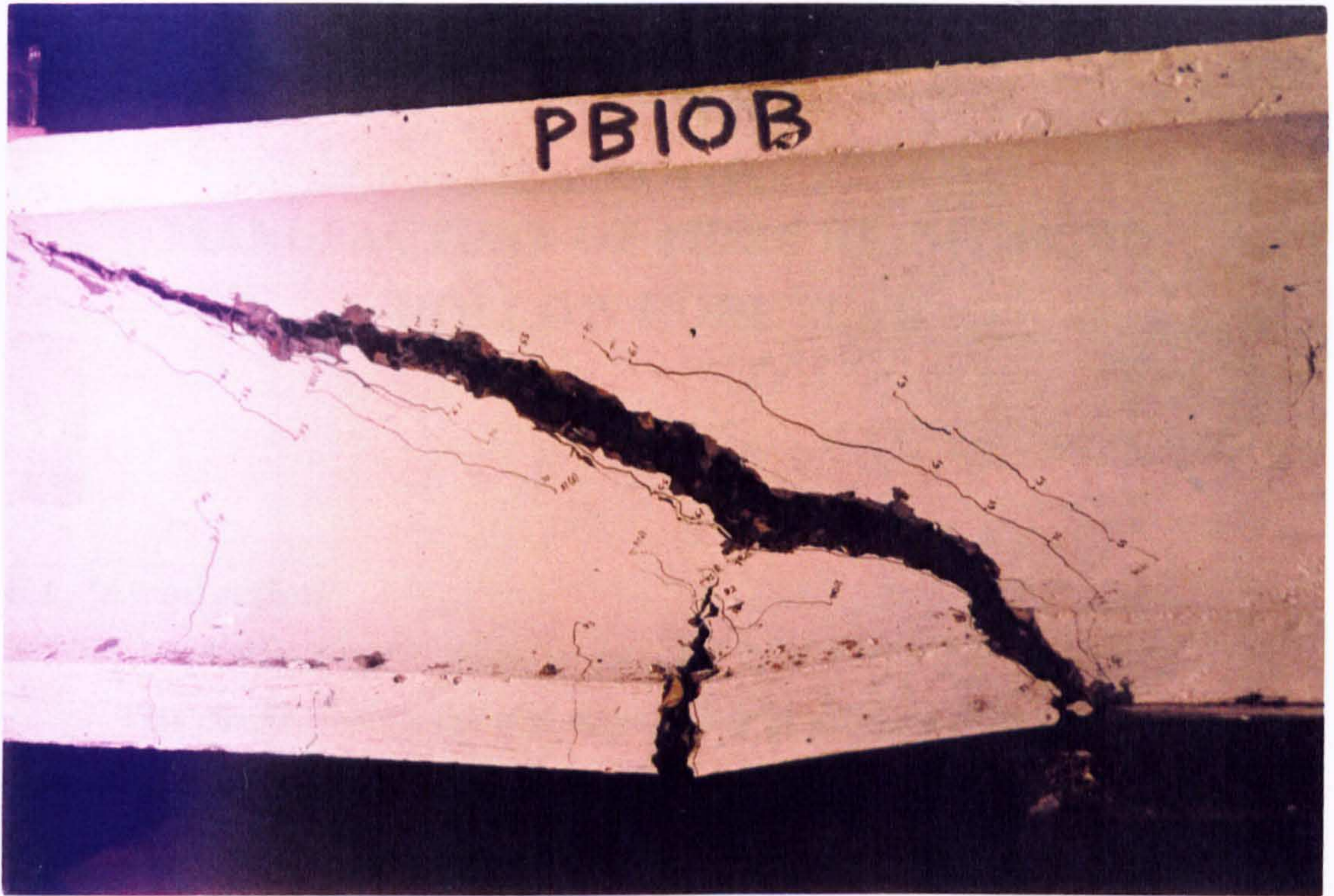
Plate 5-5 "Soffit crack" in beam PB10B
