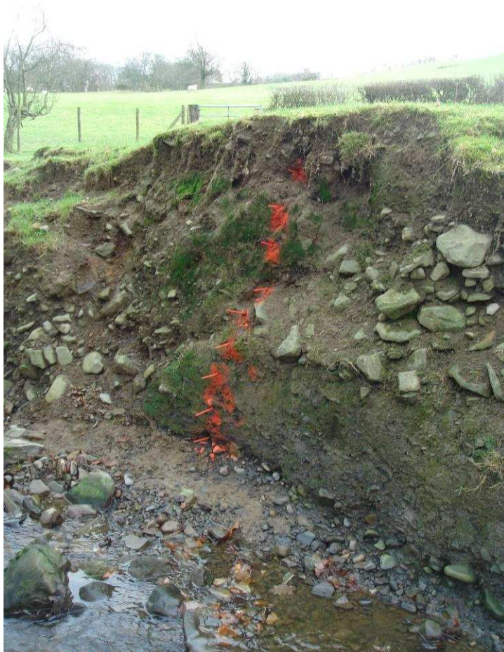
Figure 4.3 Bank erosion monitoring site 17 (Pines) on the Nant Gelli-Gethin.
