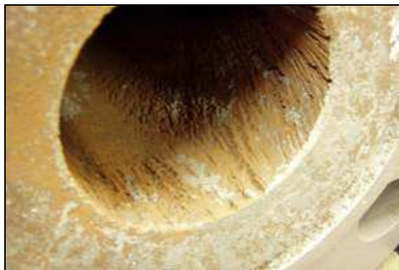
Figure 1.3: Erosion inside a steel pipe (adopted from www.aludra.nl )
