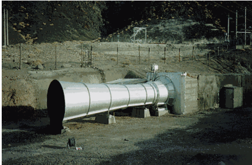
Figure 5-7: A main mine fan
