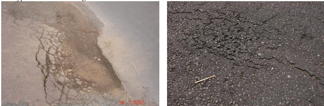
Fig. 2. Different Examples of Road Distress Types: (a) Pothole Distress; (b) Cracking Distress
