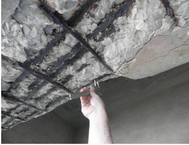
Figure 13. Diameter measurement of an extremely corroded bar.
