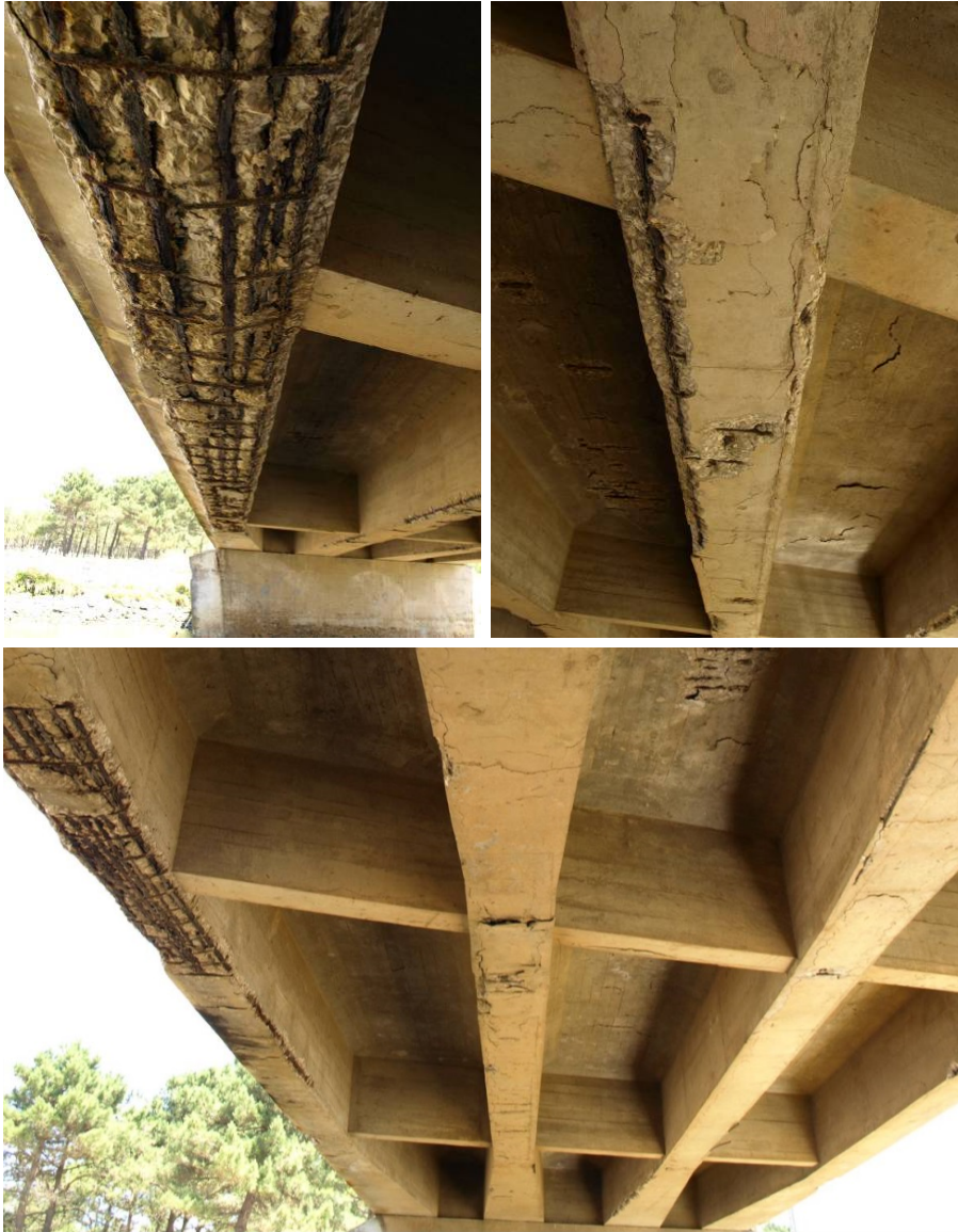
Figure 2. Deck photographs showing its deterioration state.
