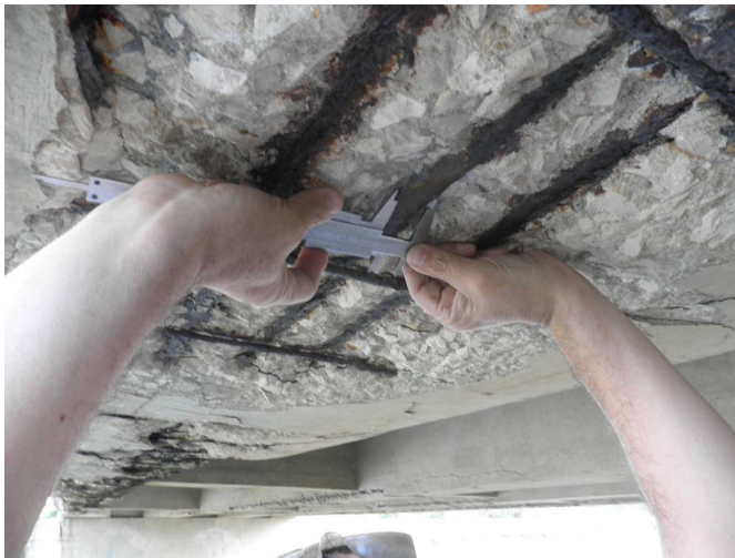
Figure 12. Diameter measurement of an exposed bar.
