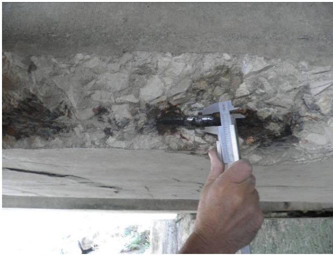
Figure 14. Diameter measurement of an edge corroded bar.
