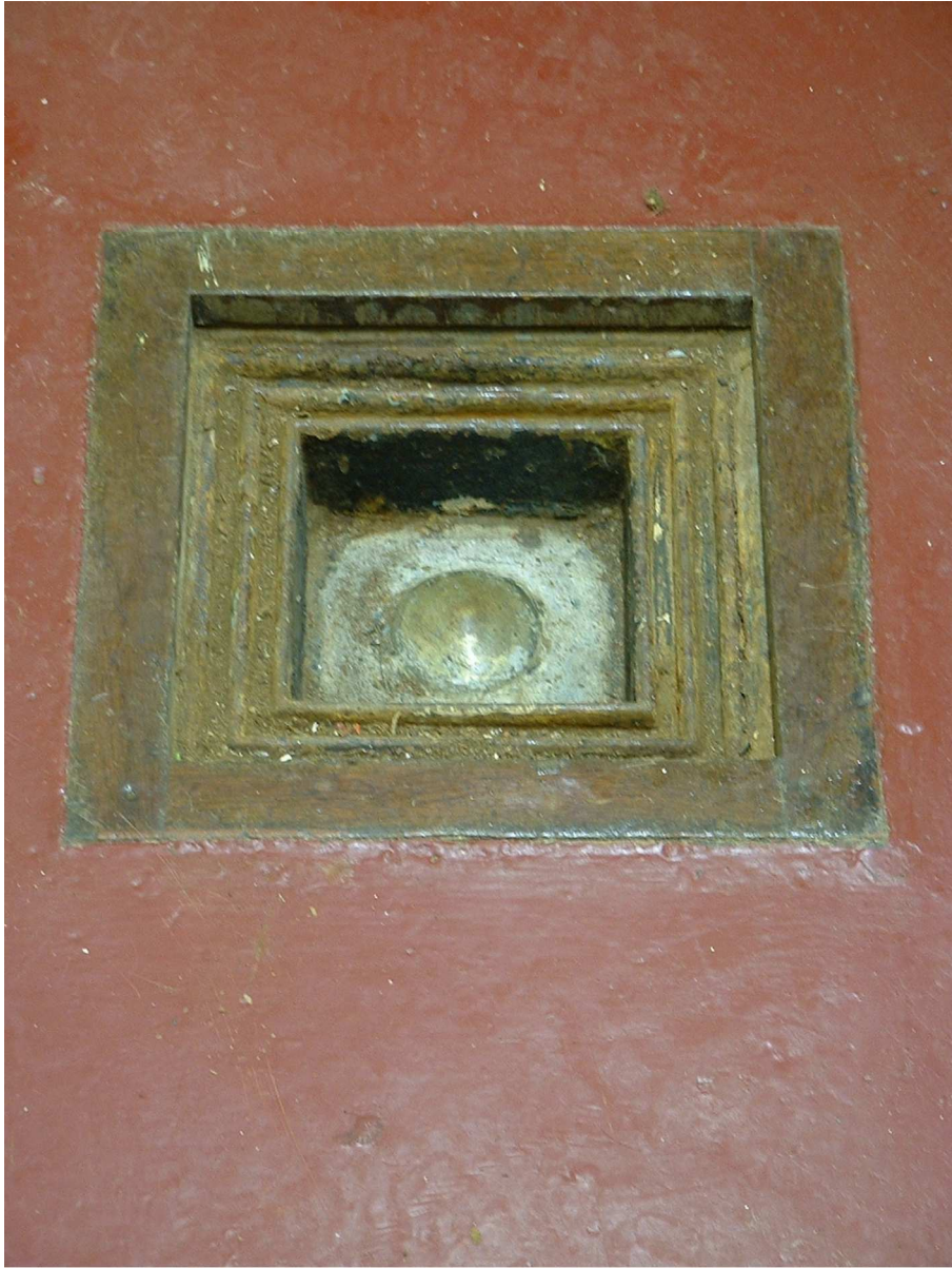
Figure 3. (a) The brass bolt benchmark (OS BM 4676 2855) which is located in the Tidal Observatory and from which the ODN national datum is defined as being 4.751 m below the mark. 423x564mm (72 x 72 DPI)
