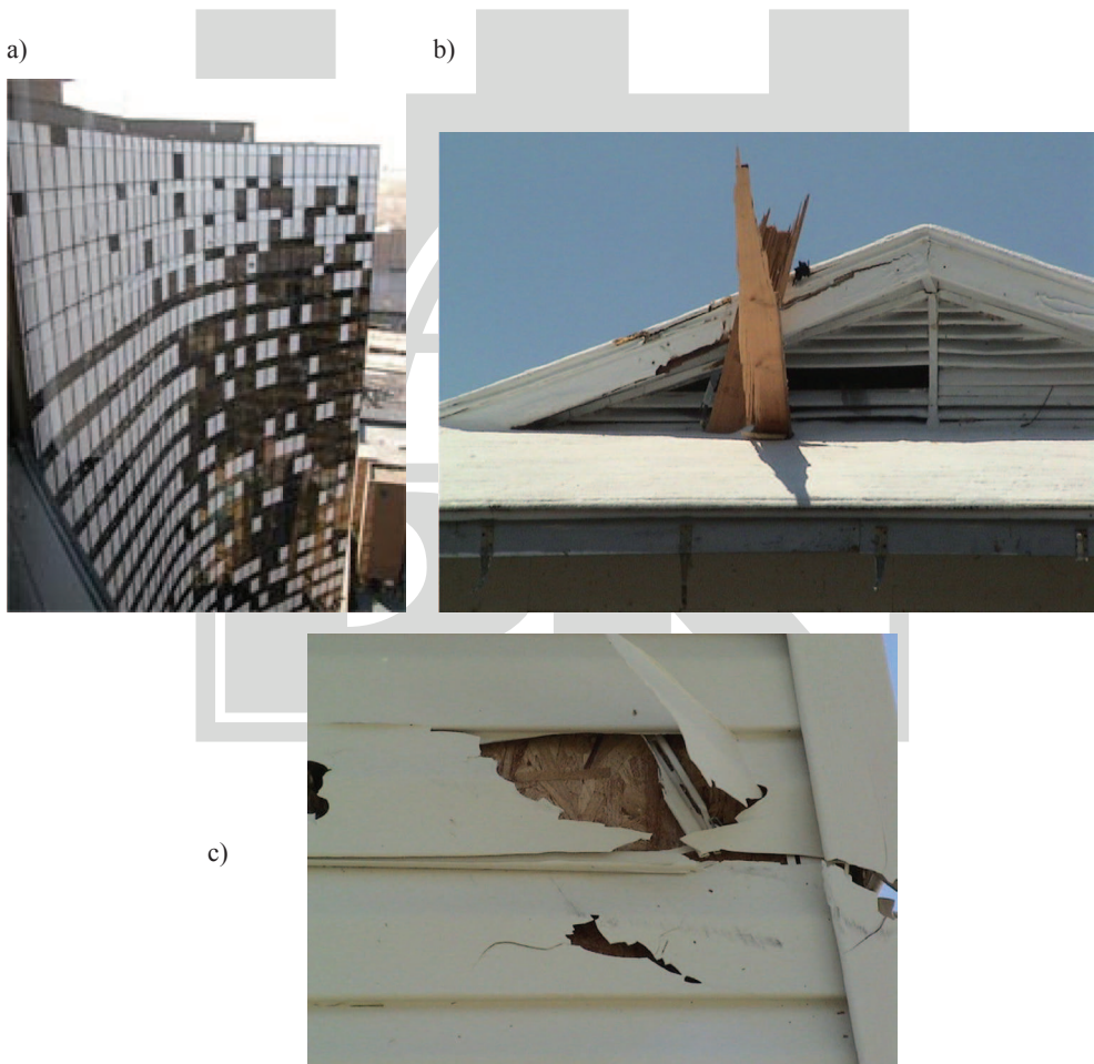
Fig. 1. Examples of damage caused by windborne debris, a) north façade of Hyatt Hotel, New Orleans damage by pea gravel from neighbouring roof (photo by K. Porter for MCEER), b) example of hazard due to missiles generated by failed structures (photo by T. Reinhold, AAWG gallery), c) example of cladding damage due to windborne missiles (photo by T. Reinhold, AAWG gallery)
