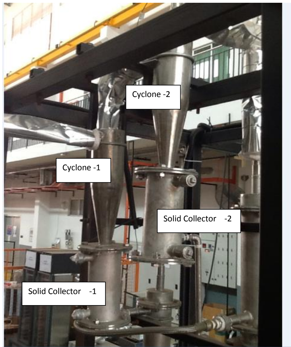
Figure 3-7: Picture of cyclone separators with solid collectors
