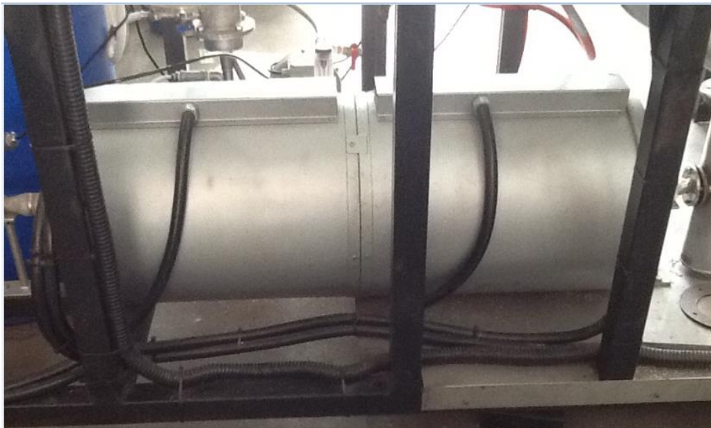
Figure 3-6: Picture of preheater
