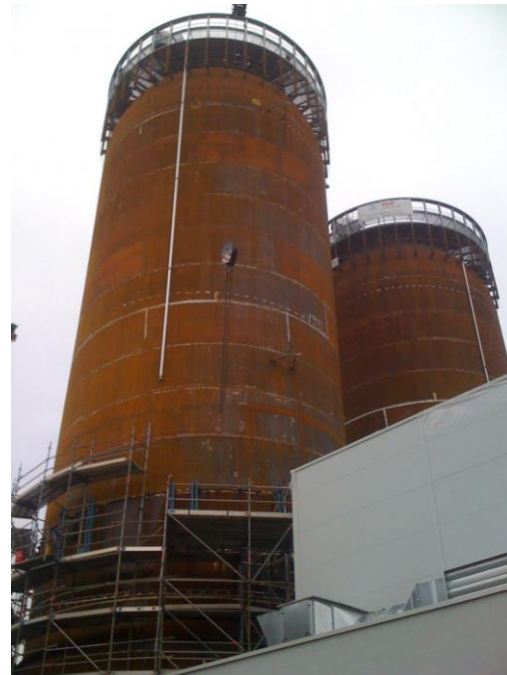
(c) Steel Tanks 8
