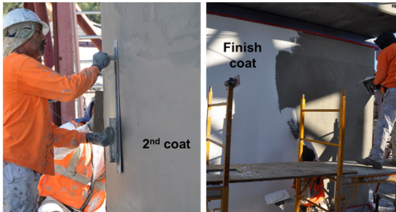
(d) Second coat and finish coat application Figure 5: Steps involved in EIFS application
