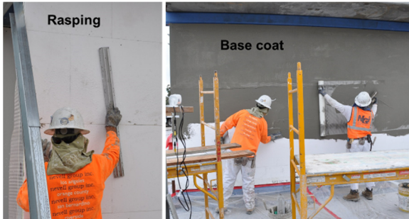
(c) Rasping of foam boards before base coat application with embedded reinforcing mesh
