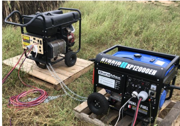
Figure 4-2: The generators used to power the LF-MRI system. The right (Duro) and left (Generac) units have ratings of 12 kW and 12.5 kW, respectively.
