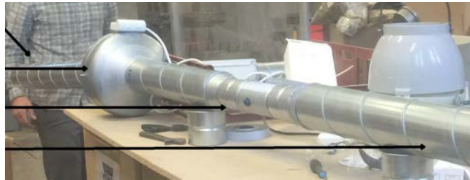
Fig. 4-30. Ventilation system before insulation
