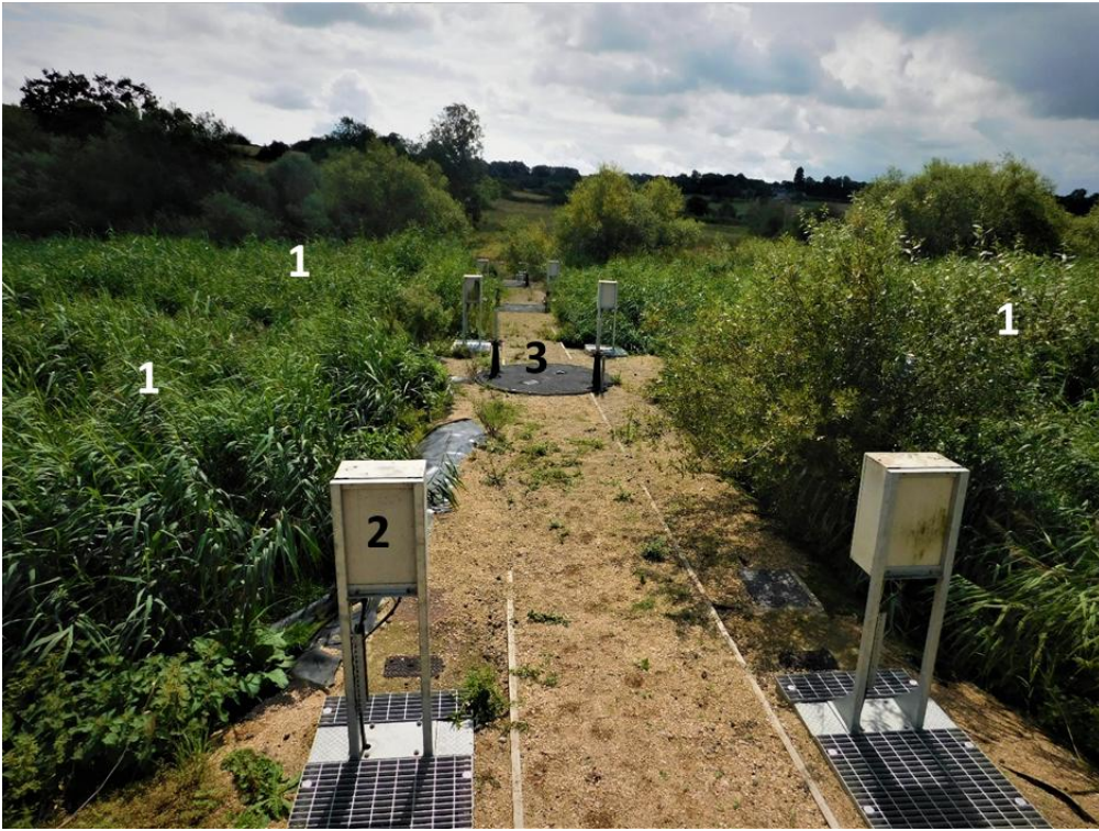
Figure 1 Gravel-Steel Slag Horizontal Flow Constructed Wetland used as a polishing step at municipal wastewater treatment plant, Devizes, Wiltshire, UK. Effective operation of treatment cells (1) is ensured by flow meters (2) synchronized with separated distribution chambers (3). (Photo. F. Bydalek)
