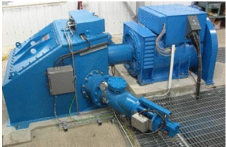
Fig. 4 Typical single-jet Turgo turbine installation, with inlet pipe under the powerhouse floor [2].
