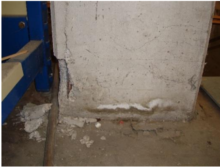
Figure 3. Damage at the column base after the event on May 29 th
